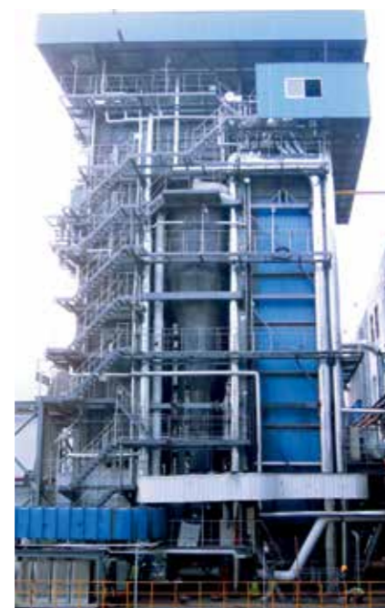
山东兖州 75 吨 / 时高温后燃循环流化床锅炉 75 t/h CFB Boiler with High Temperature and Post-Combustion in Shandong Province
